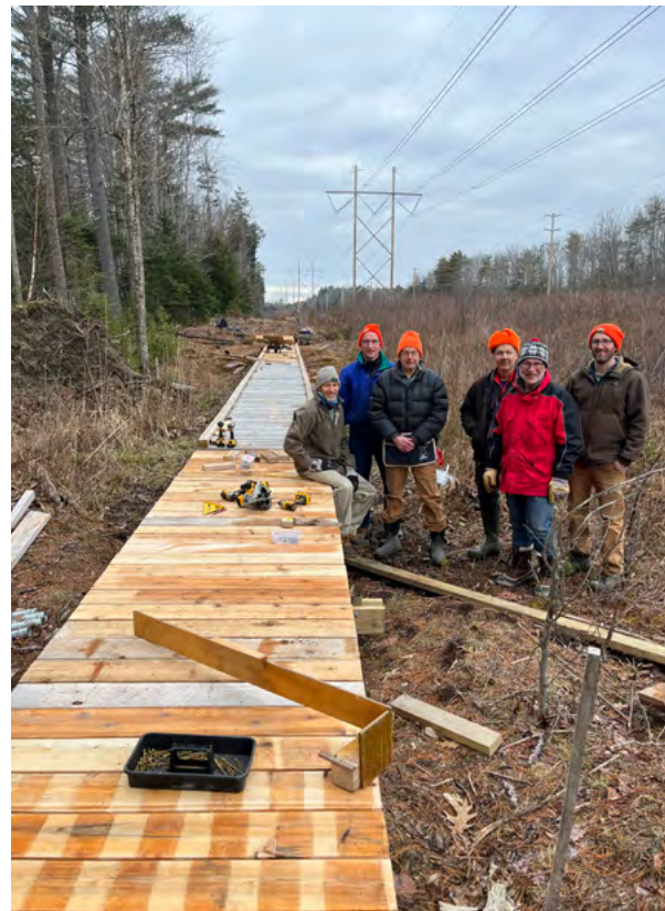
Building the last mile of the West Side Trail Photo: Yarmouth Community Services
