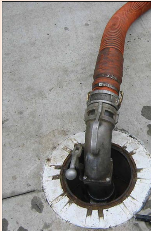
Delivery hose hooked to the fill pipe in the spill bucket.
