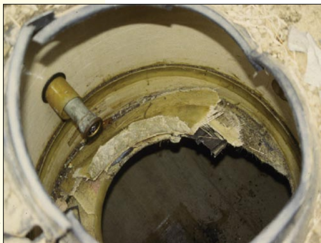
A manway opening that blew open as a result of a pressurized delivery made to a tank equipped with a ball-float valve.
