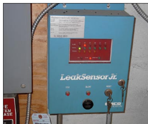
A leak sensor in alarm.
