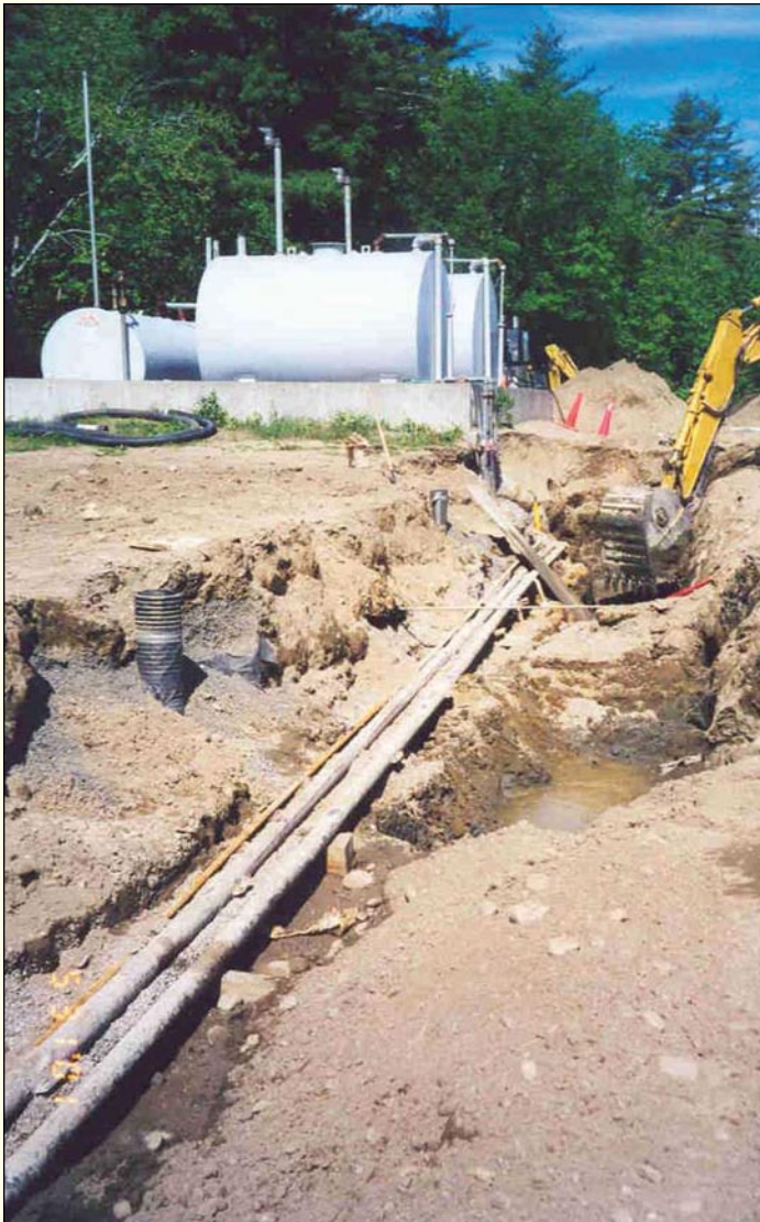
Underground piping associated with ASTs is a frequent source of leaks.
