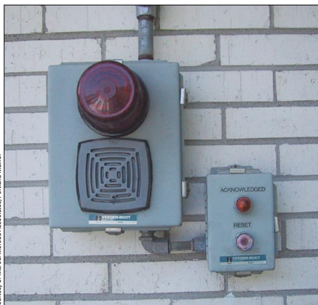
This is a typical unlabeled overfill alarm. These alarms should be labeled so the delivery driver knows where it is and what it is.
