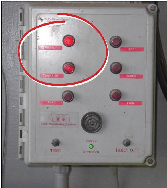
A tank interstitial leak sensor in alarm.
