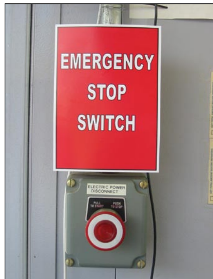
Courtesy of Marcel Moreau Associates, Portland Maine.
