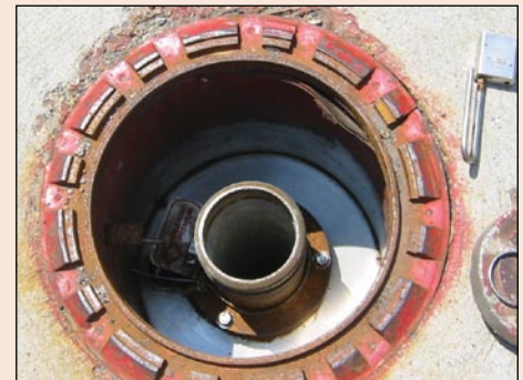
Below-grade spill bucket.
