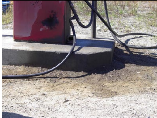
Spills to gravel.
