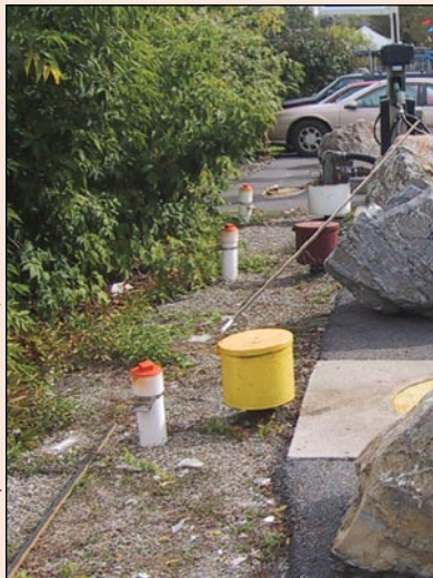
Above-grade spill buckets.
