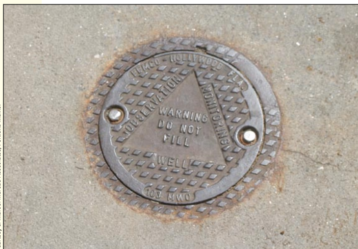
Courtesy of Marcel Moreau Associates, Portland Maine
