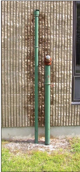
Overfill spill into soil.
