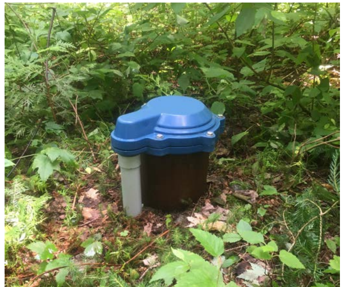
Wellhead with a sanitary seal, Poplar Stream Falls Hut
