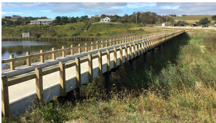
FIGURE B.2 - Single-lane bridge on piers in Chilmark, Massachusetts, that spans an area projected to flood more frequently with sea level rise. Photo by Slade Moore.
