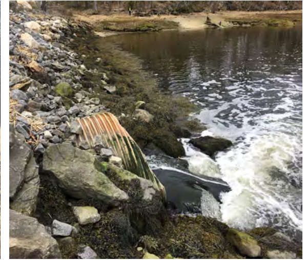
FIGURE 1.8 - This perched, undersized culvert blocks aquatic organism passage except during high tide. Photo by Slade Moore.
