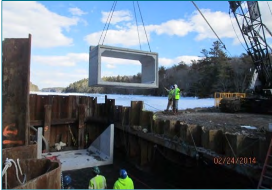
FIGURE B.8 - Maine DOT installation of precast concrete box culvert with twelve-foot span and six-foot rise. Long Reach Lane, Long Marsh, Harpswell, ME. Image source: Casco Bay Estuary Partnership.
