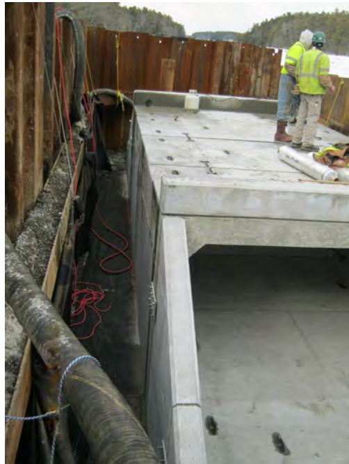
FIGURE 8.2 - A sheetpile coffer dam was utilized to isolate the work area from tidal flows during the replacement of the Long Reach Lane tidal crossing in Harpswell. Photo by Charlie Hebson.
