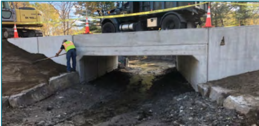
FIGURE B.5 - An embedded pre-cast concrete box culvert, with 16-foot span by 8.5-foot rise. Lubberland Creek, Newmarket, NH. Image source: Peter Steckler.
