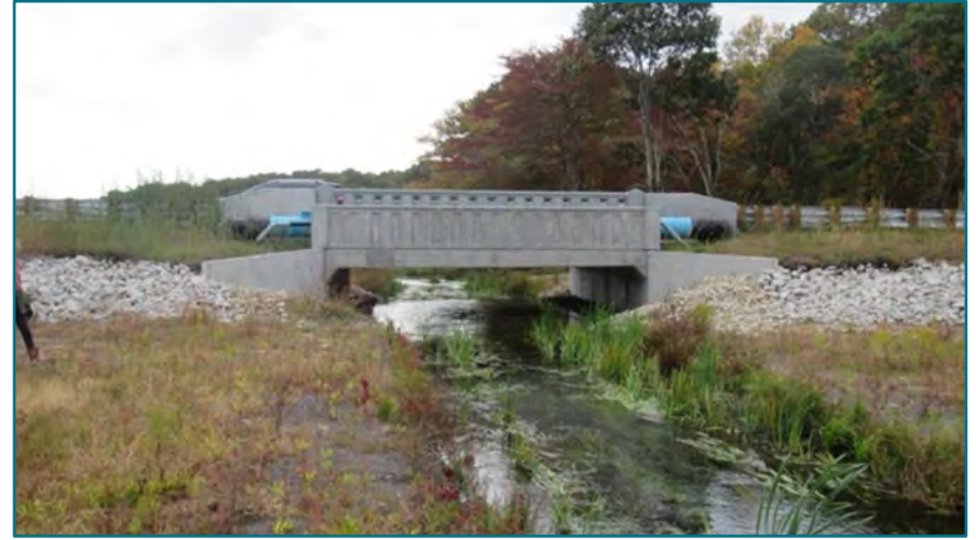
FIGURE B.6- A three-sided concrete rigid frame structure, installed on pre-cast footings. Clear span of 24 feet. Structure includes a pre-cast modular design with six-foot-long sections. Due to cover limitations within the road prism, an insulated water line was attached to side of headwall. Coonamessett River, Falmouth, MA. Image source: Inter-Fluve.
