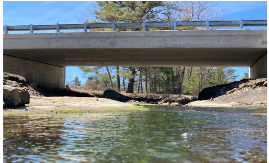
The sequence of best practices encouraged by the CoastWise Approach encourages the development of safe, climate resilient, cost-effective, and ecologically supportive crossings. Photo by Slade Moore.
