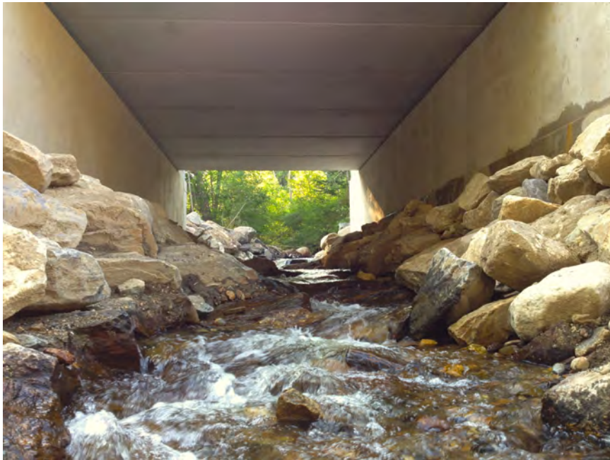
FIGURE 5.3 - This MaineDOT crossing was designed to adequately accommodate storm flows, protect footings from scour, facilitate low-flow water depths sufficient for fish passage, and allow for semi-aquatic wildlife movements. Photo by Slade Moore.
