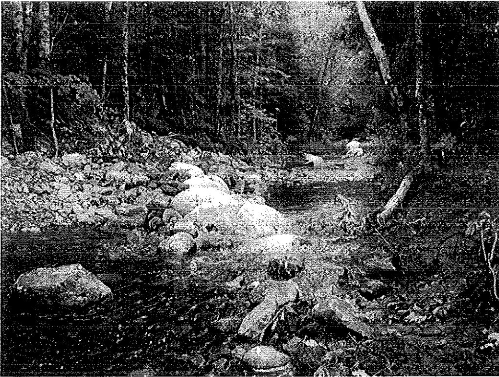
Rock sill, East Branch Enchanted Stream, constructed 2008 to encourage meander development and to scour pools.
